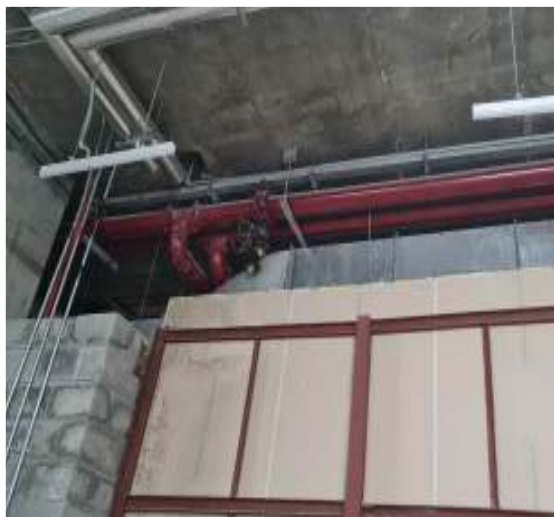
Space equipped with Fire Fighting Lines / FHC
